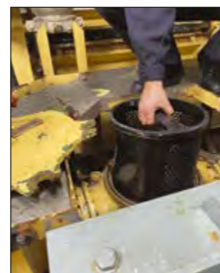
Fig. 3: Additively manufactured filter insert of the sea cooling water system being used on frigate SACHSEN. Only feasible using level 2 3D printers because of the size
