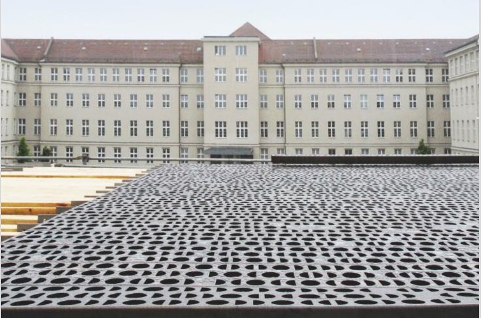
At the Bendler Block: the arrival of the bronze shell marks the beginning of the decisive construction phase.
